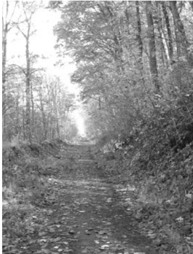
An existing rail bed in Palmer Township proposed to receive improvements and become a multiple use recreation greenway trail.
