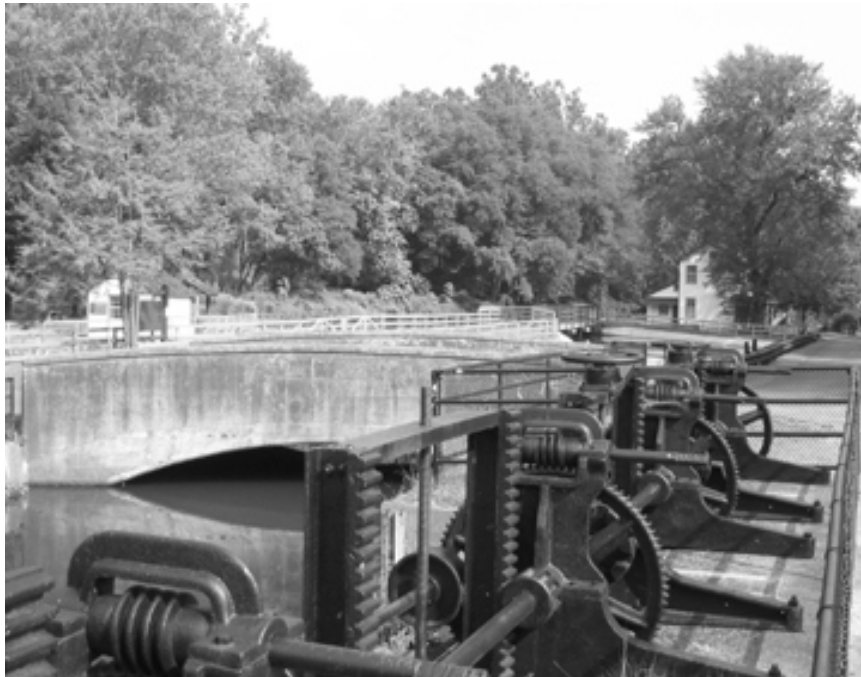
These mechanisms opened and closed this lock chamber on the Delaware Canal near Raubsville.
